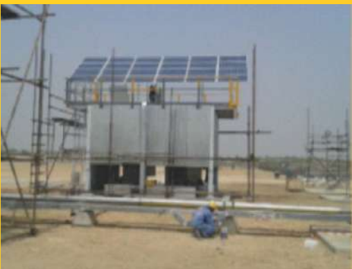
▶ Control Panel Shed
